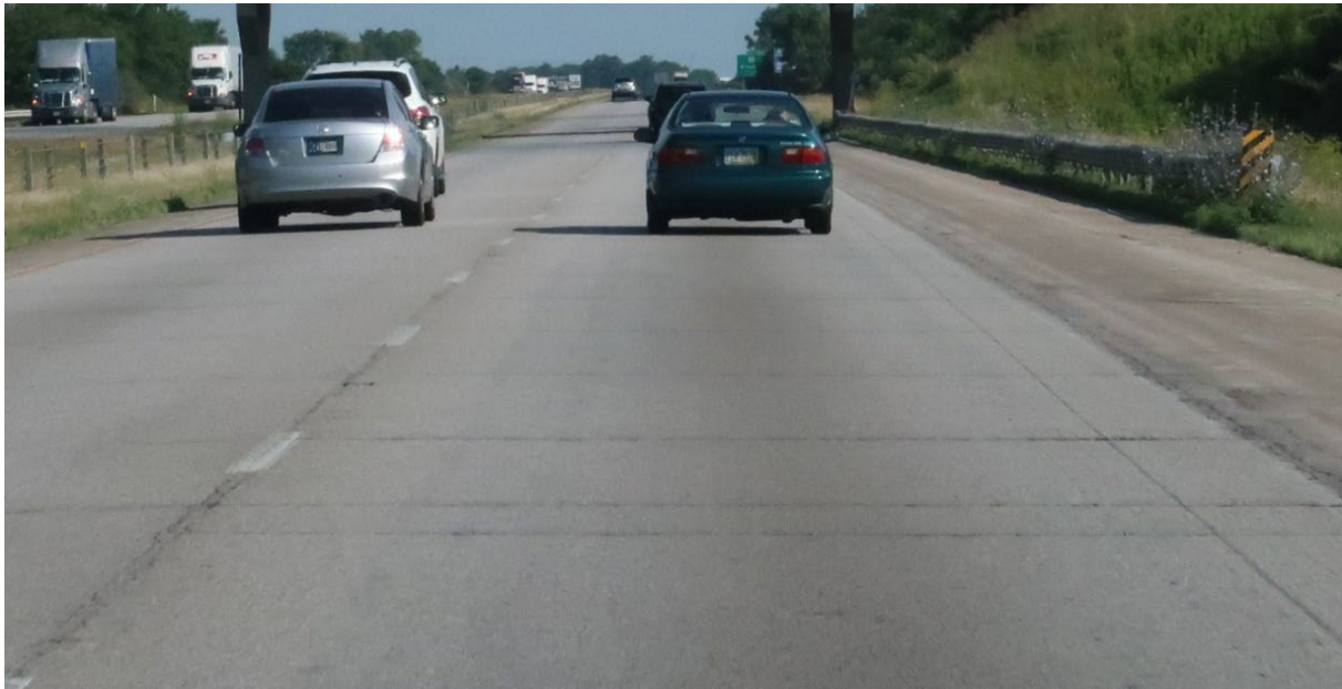
Roadway with worn pavement markings
