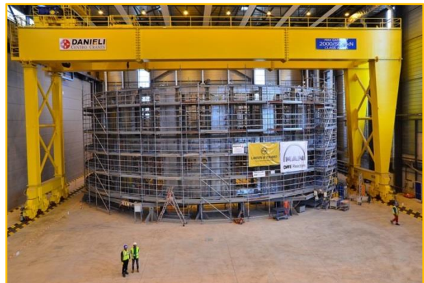
FIG. 8: The ITER scale is apparent in the Cryostat Workshop, where Larsen & Toubro is supervising the assembly and welding of the lower cylinder.
