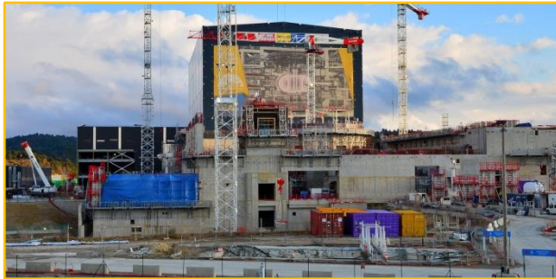
FIG. 1: A view of the Tokamak Complex with the Assembly Hall to the back. The Tokamak Pit is in the centre, the Tritium Building on the left and the Diagnostics Building on the right.
