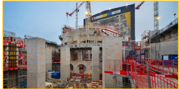
FIG. 2: The bioshield is now finalized. Openings in the wall are for cryostat bellows that will connect the machine to the port cells to give access to systems such as remote handling, heating and diagnostics.
