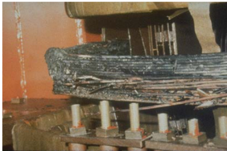
A damaged transformer at the Salem Nuclear Plant. (Metatech)
