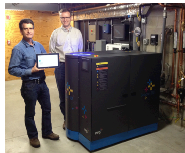
Figure 3: Example of an advanced CHP system developed by Dean Kamen of DEKA Research and Development. (Photo by G. Morgan.)
