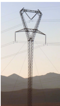
Figure 2: Example of a guyed transmission tower. Such towers can be less expensive but subject to “domino collapse.” Image from Wikimedia.
